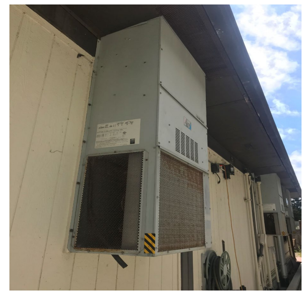
SKY B3 Portables and B21 have local Air Conditioning Units
