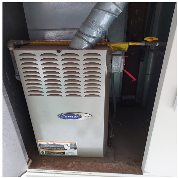
B14 and B19 have local Furnace units that provides filtered outside / indoor air that can also provide heat when called upon.
