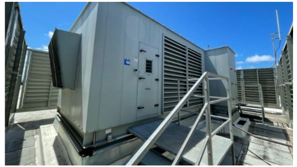
Cañada College Building 9 AHU-1
